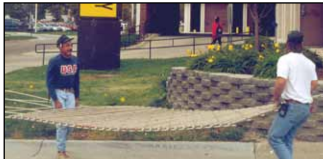
Figure 11.1: Large sections of preassembled formwork can be installed with ease (courtesy Vector Construction Group).
